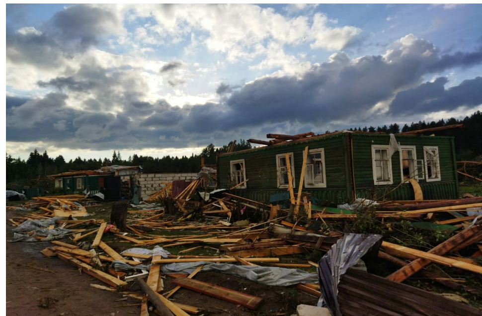
Tornado-induced damage in Andreapol town [ https://vk.com/meteodnevnik ]
